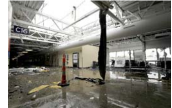
Tornado damage on Lambert's C Concourse. Photo: OneTravel.com
